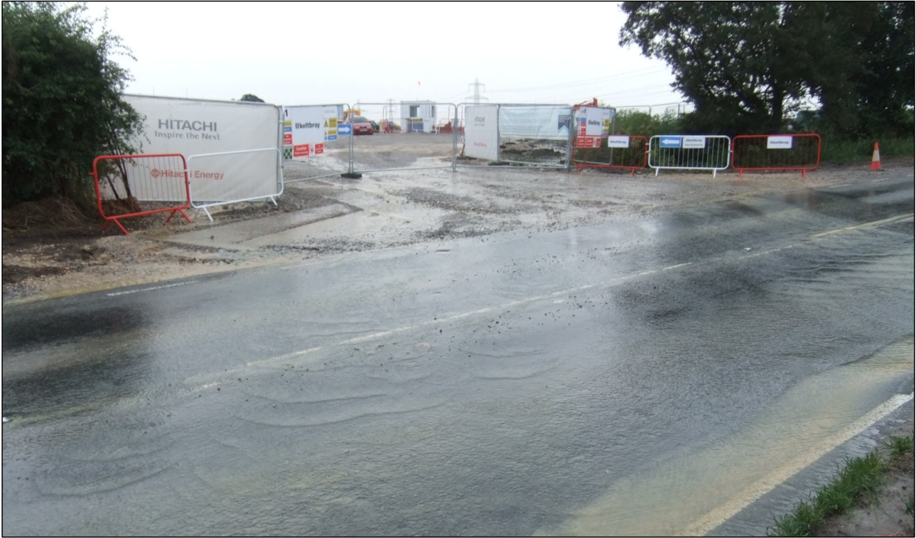
Figure 5: Hornsea Three onshore substation site entrance
